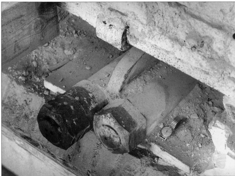
Fig. 18 Neues Museum, Room of the Niobides, end of bowstring girder, connection between wrought iron tie rods and cast iron arch (photograph 1993, W. Lorenz)
